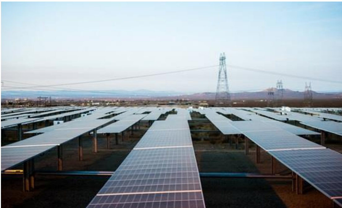
Figure 10 Solar panels producing renewable energy at the Pearblossom solar facility 2018
